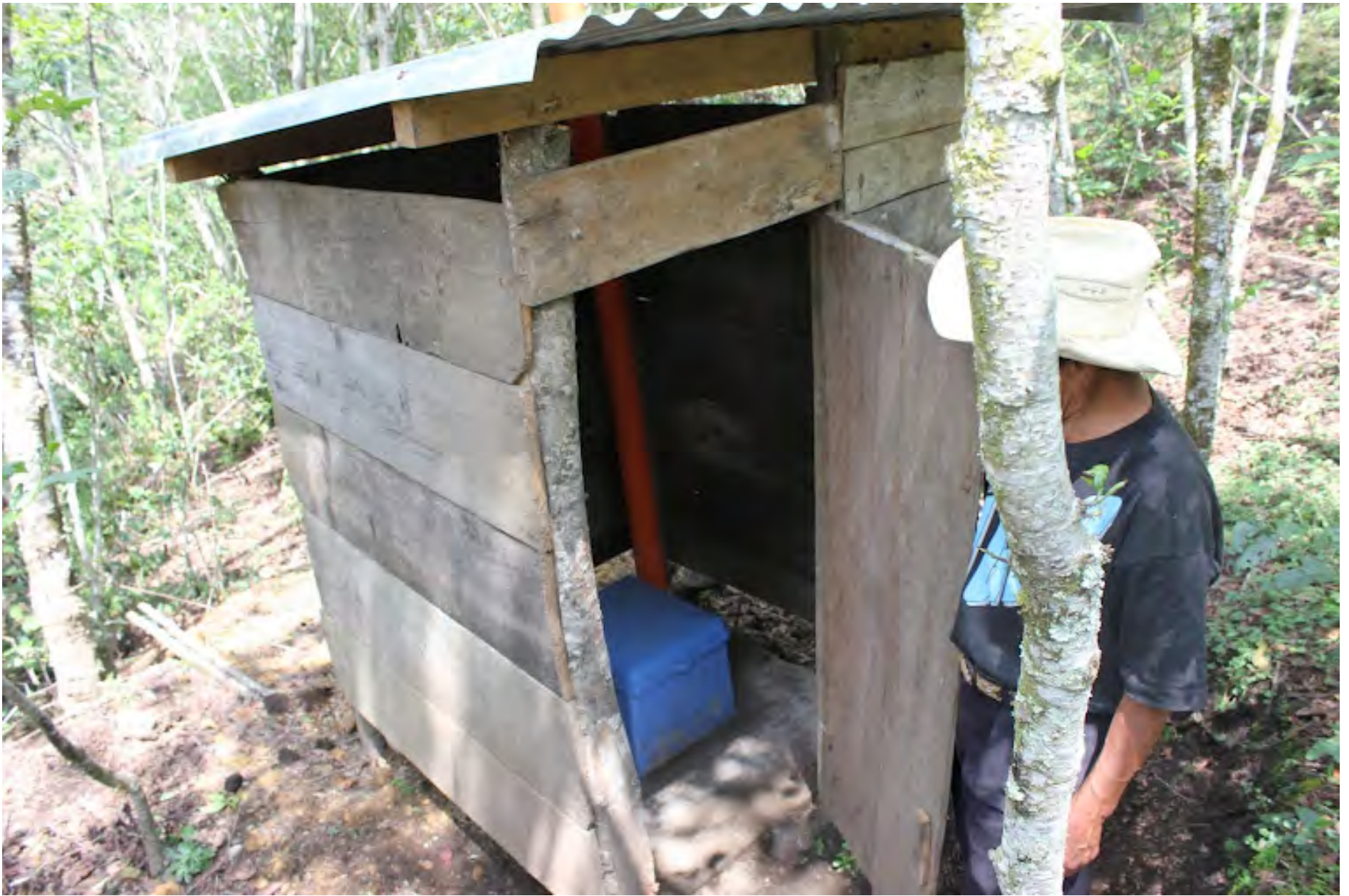
Installed Latrine – Concrete base, toilet with closing lid, sturdy construction, vented
