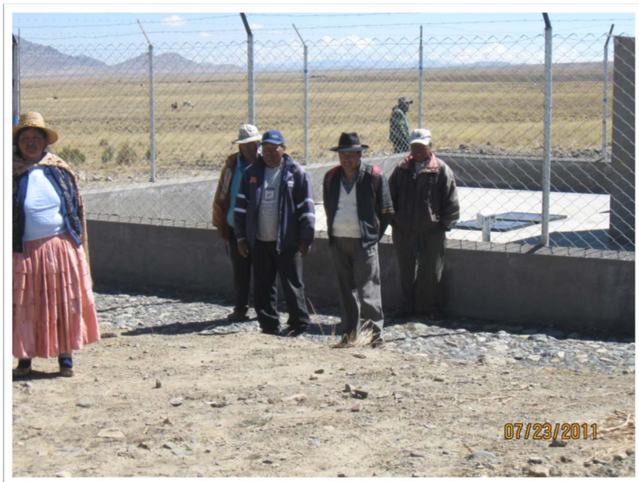
Figure 9 - Machacamarca water storage tank with security fence
