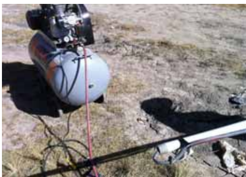
Equipment needed for air developing a water well - 1" PVC with air insert - to draw out fines
