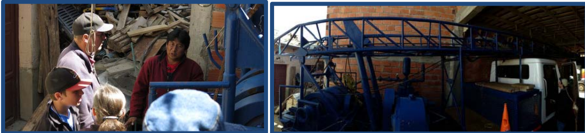
R-Jaime explains the many improvements Suma Jayma has made to the rig. R-The water well drilling rig
