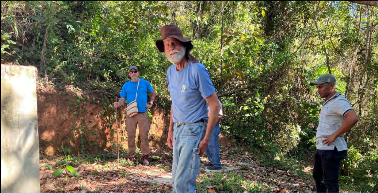
The WEFTA team reviews the new tank construction (performed by Nicolas and Cheo) in the community of Zapote. Due to the drought, the new water storage tank is dry.
