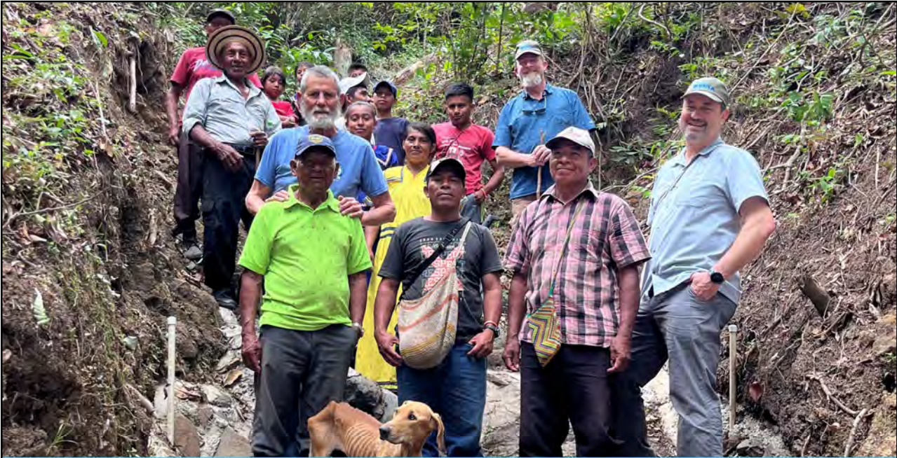
The WEFTA team and Nicolas with the water committee of Llano Majagua standing on the newly constructed spring capture that serves the community.
