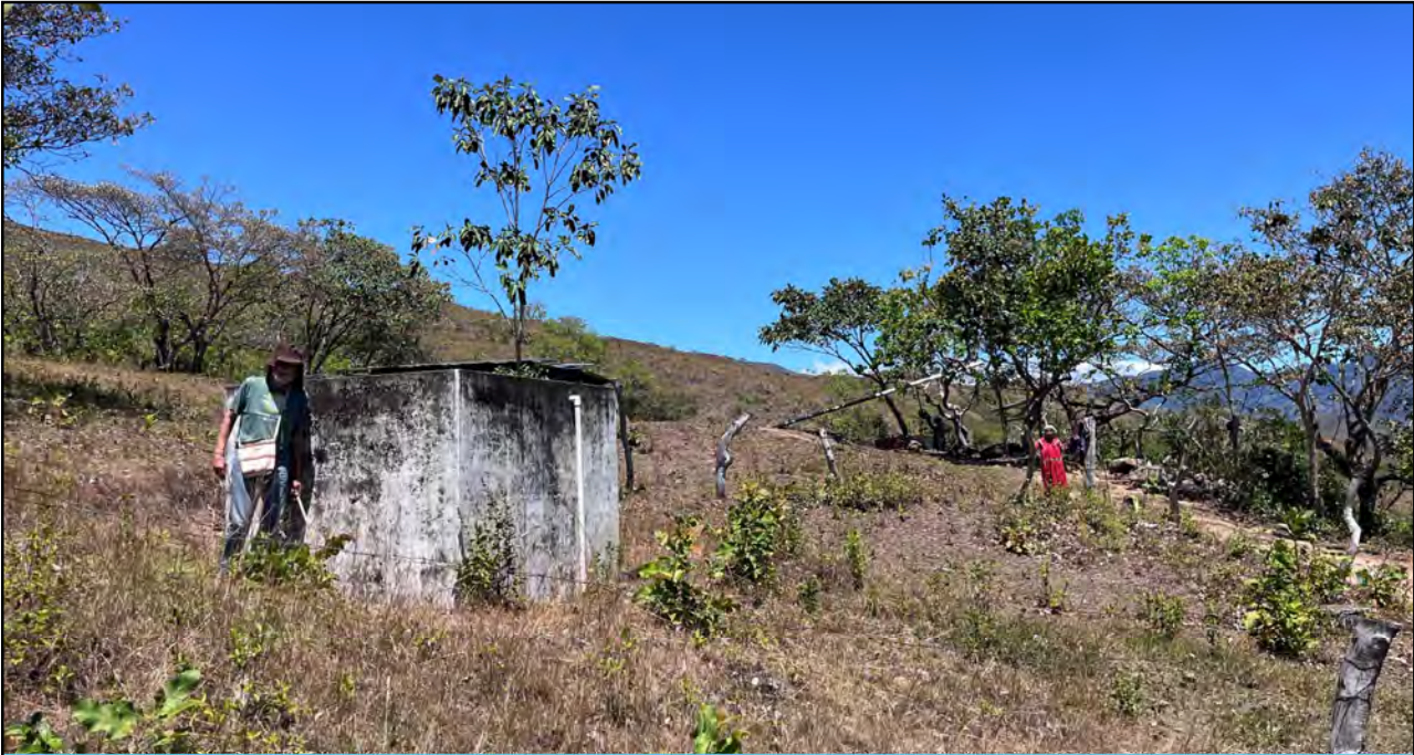
WEFTA Volunteer, Father Robert, assesses the condition of the water supply tank of the community of Cerro Grande.
