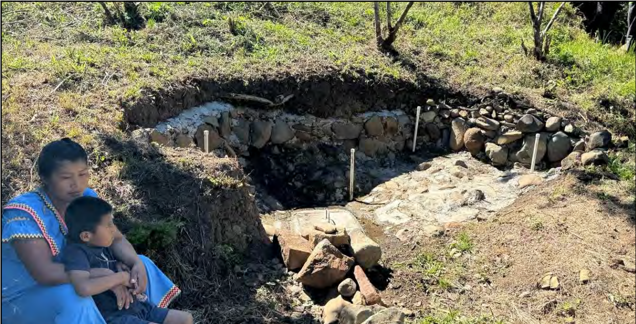
An Alto Majagua community member and child sit near the newly constructed spring capture for the community of Alto Cienega.
