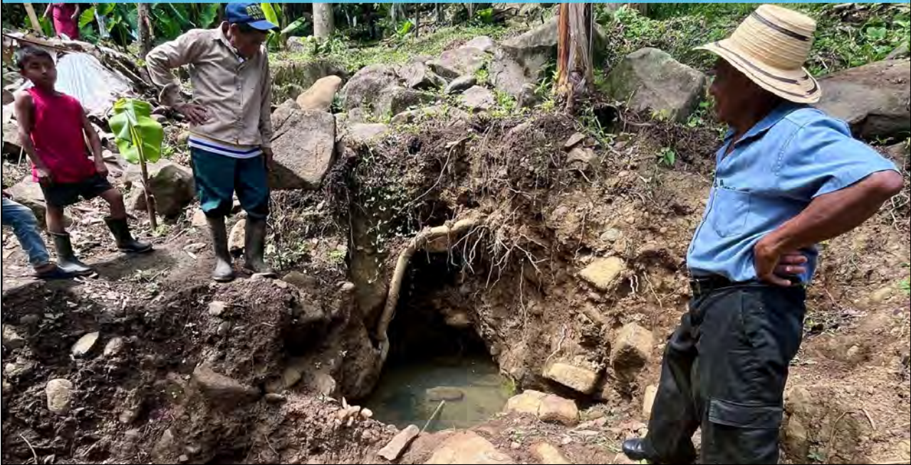
The WEFTA team assesses a new spring source for a family in Valle Risco. The spring source will be protected using rock, gravel, and cement mortar to allow the water to flow out of the spring in pipe without any contamination from the surface.
