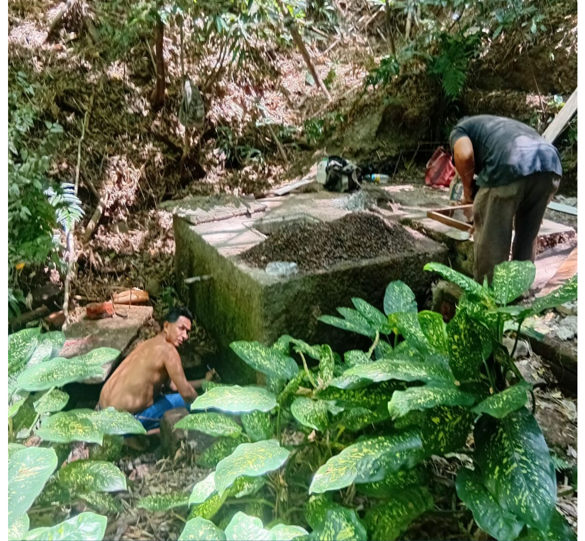
Water committee and community members work to clean the spring box gravel filters and clean the area where spring water enters the spring box.
