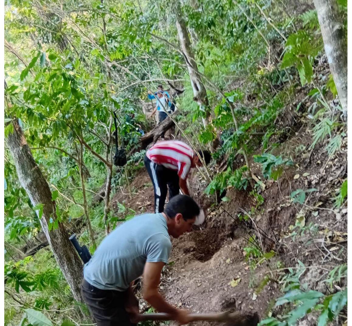
Tree roots and land movement made repairing the transmission line imperative. Digging through the area was not easy either!
