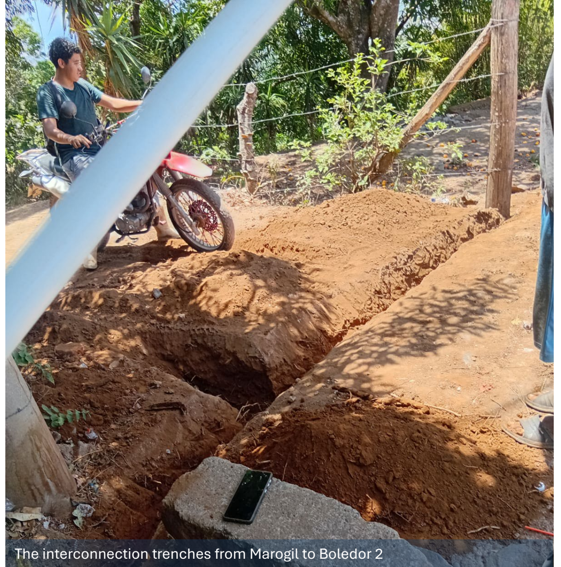
The water distribution line for the Marogil system runs parallel with the excess water line running from the Marogil storage tank to the Boledor 2 storage tank.
