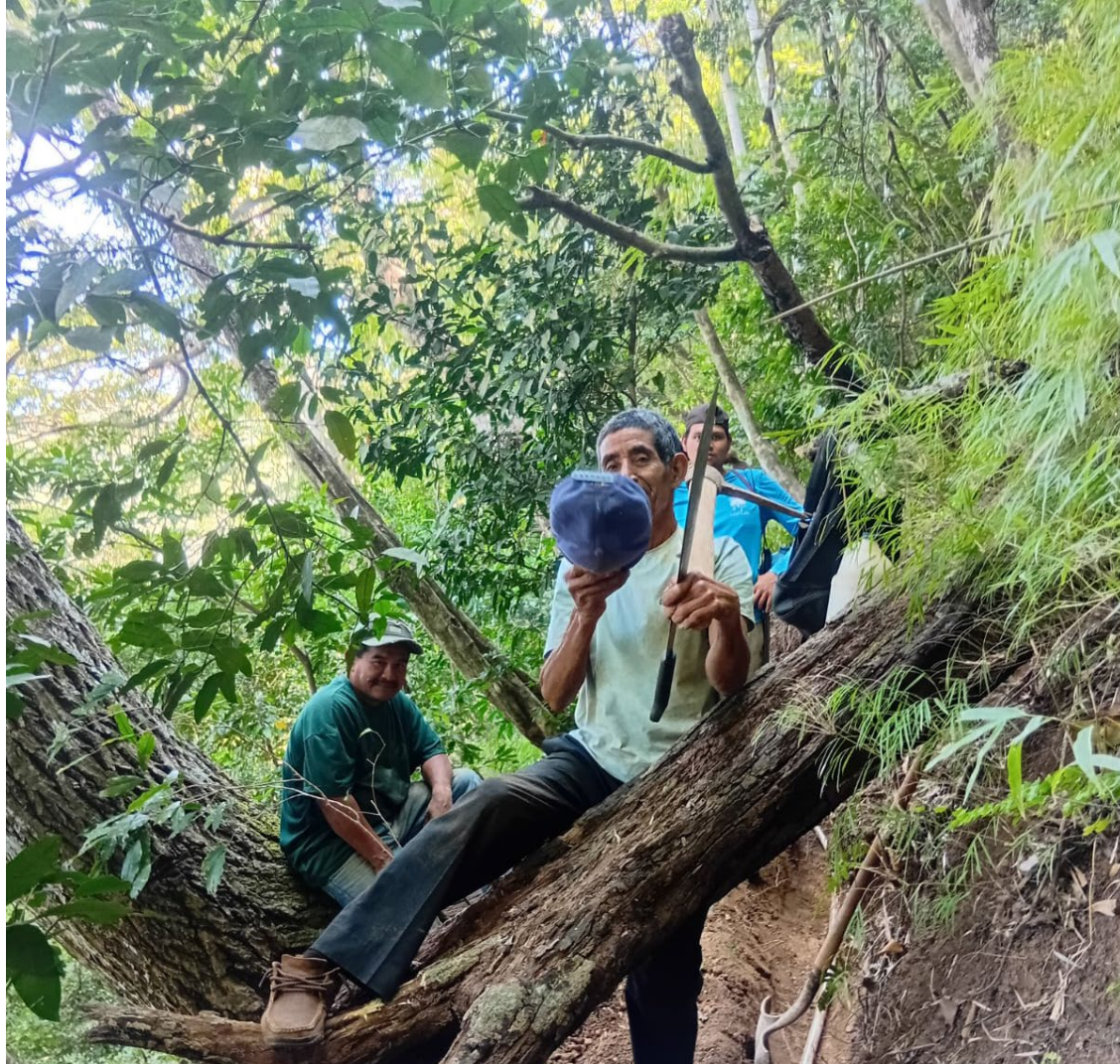
Water committee and community members dig to repair and replace portions of the transmission line from the Marogil Spring to the water supply tank.
