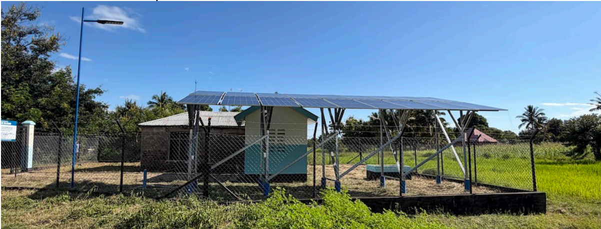
Lituhi Solar pumping system
