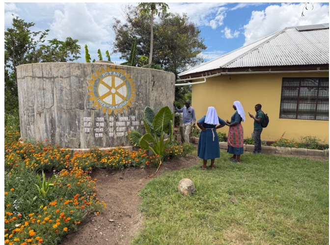
Nonfunctional rain water harvesting tank - needs repair
