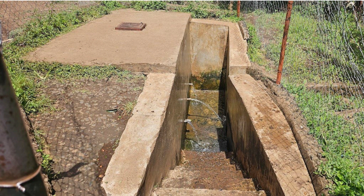
Protected spring at Kemchange –community need to replace taps to reduce water wastage
