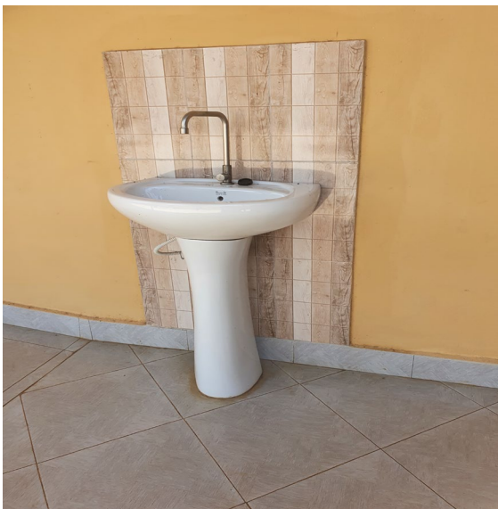
Dry handwashing basin at the Baraki HCF
