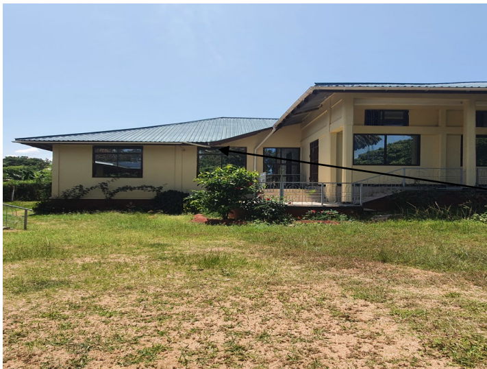
Broken gutters at the conference hall
