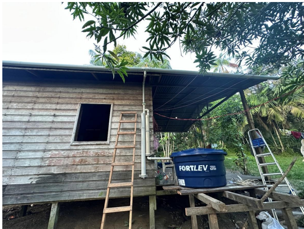
Image 1.12. Filtering system and connection to the storage tank, Villa Olivença.
