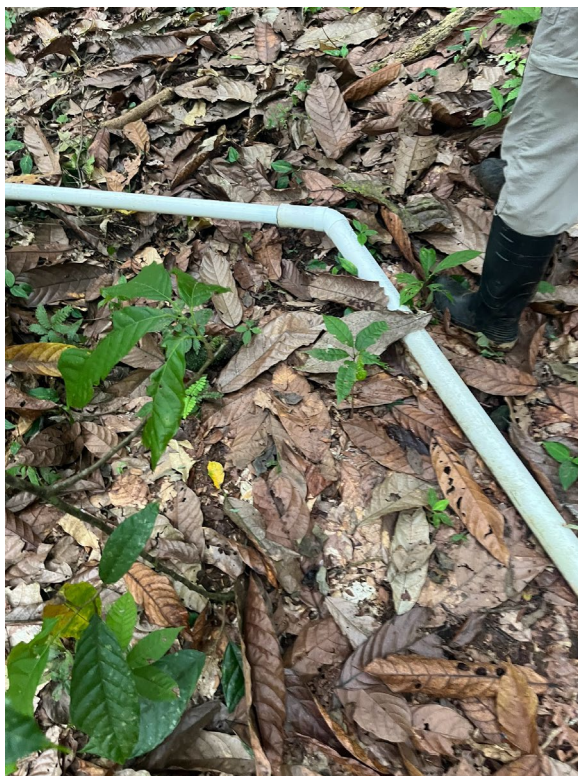
Figure 38: Rio Oeste Pipe Elbow
