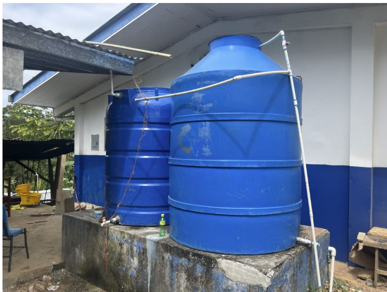
Figure 31: Temporary School Tanks
