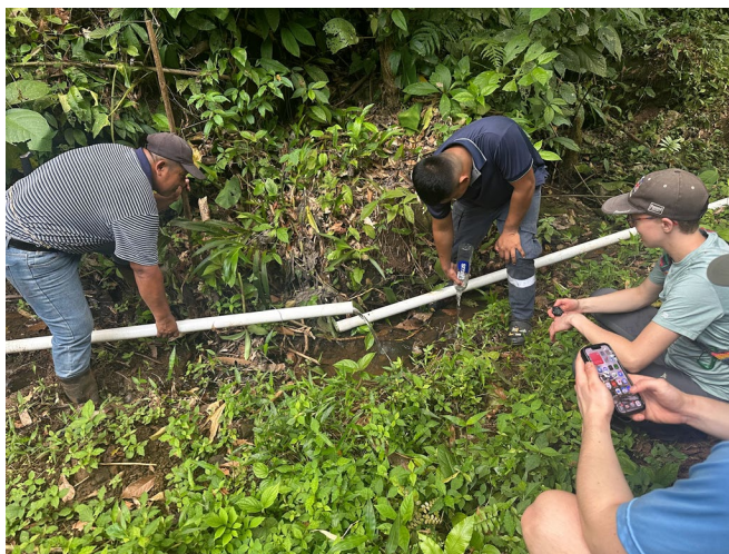
Figure 35: Flow Rate Testing at Rio Oeste
