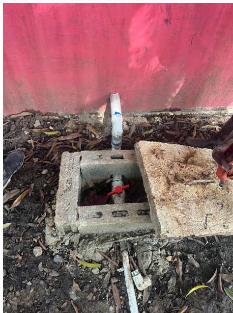
Figure 21: Carrisal tank intake, valve half open to control flow
