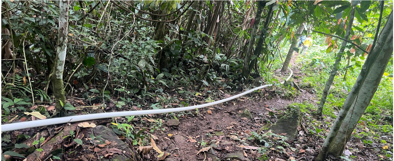
Figure 12: Mario Lopez Arriba Pipeline
