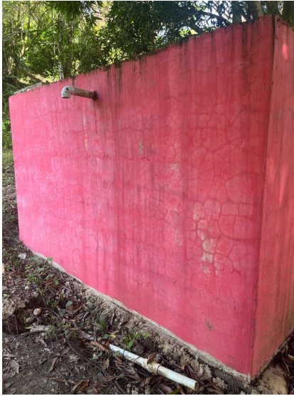
Figure 19: Carrisal tank cleanout and overflow
