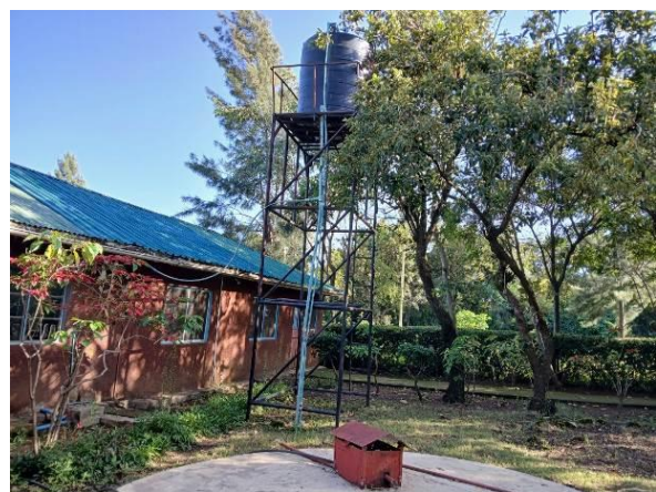
Existing storage tank 2000L on 6m tower
