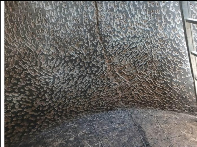
Observed cracks in the tank walls
