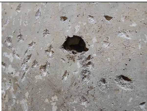
Observed holes in the tank walls
