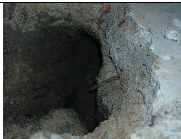
Observed holes in the base floor
