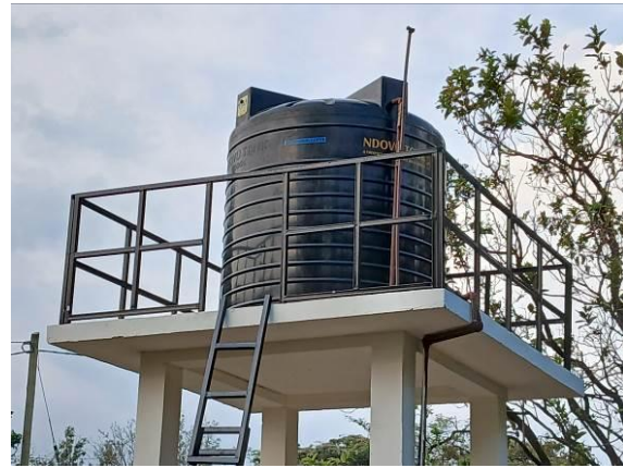
Installed tank 5000L
