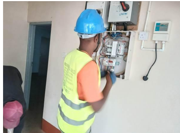
Electrical connection of solar water heater
